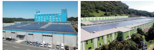
Solar Panels installed at Kumamoto Plant (left) and Kumamoto East Plant
